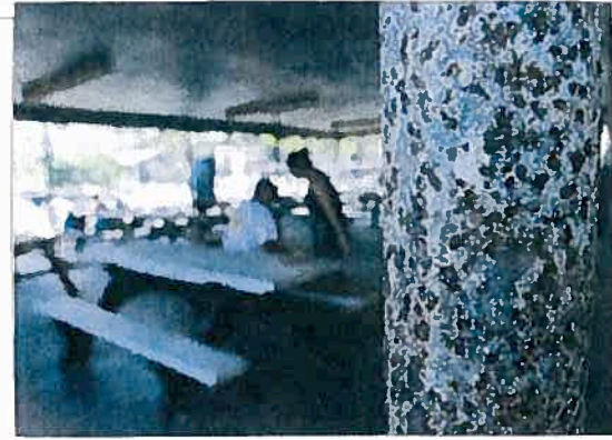
One of the rusted support poles holding up the Kahaluu Beach Park pavilion. - Photo By Baron Sekiya | West Hawaii Today
